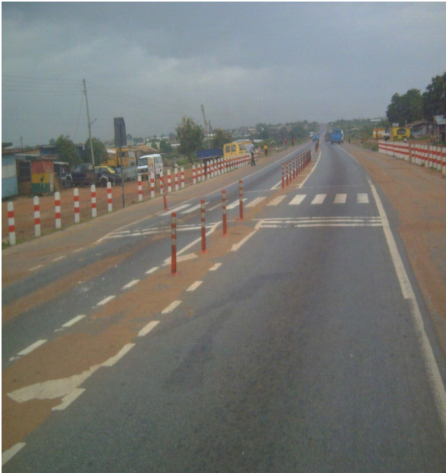
Carriageway narrowing, delineators and speed humps
